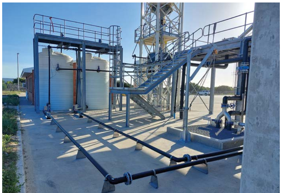
At its processing plant in Gqeberha, Eastern Cape, San Miguel has implemented advanced wastewater treatment technologies to meet efficiency, safety, and sustainability goals.
