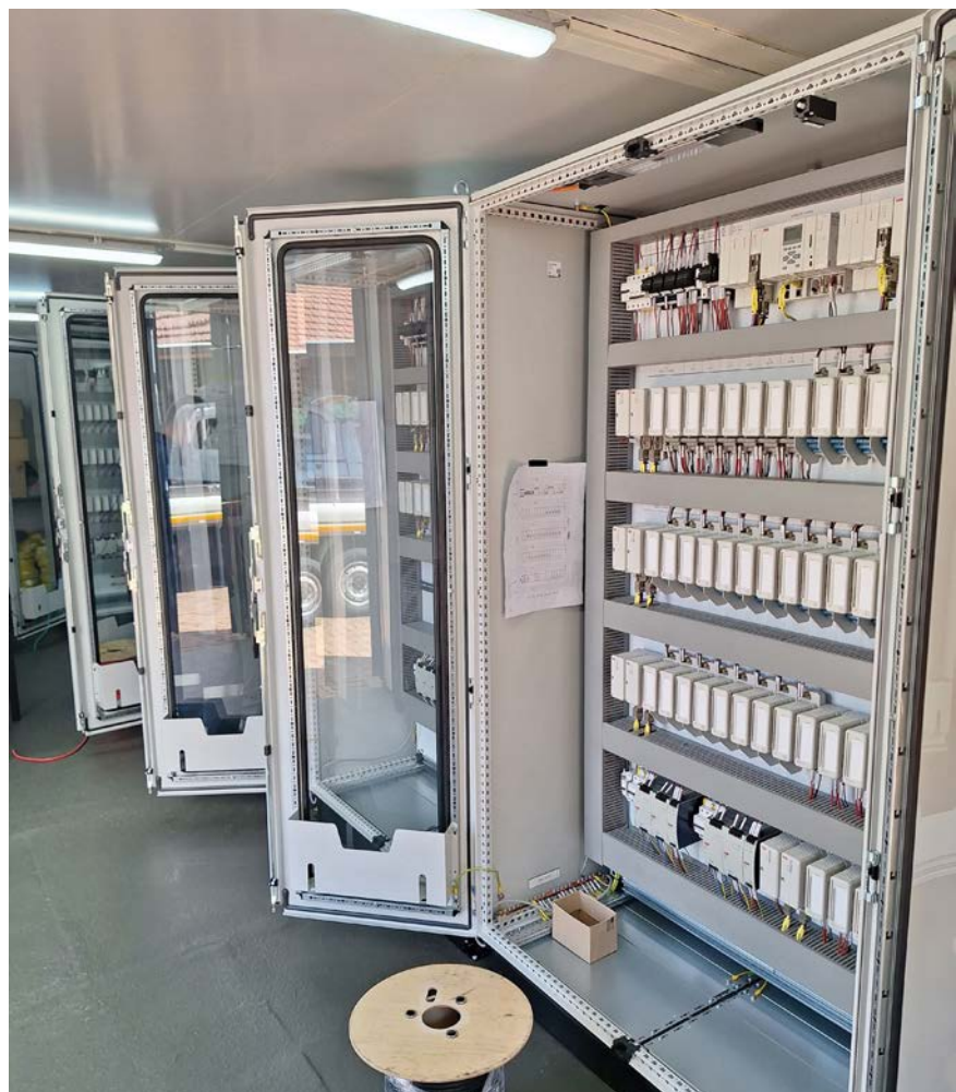
In this upgrade of the DCS, the rewiring of panels involved 12 000 I/O points.
