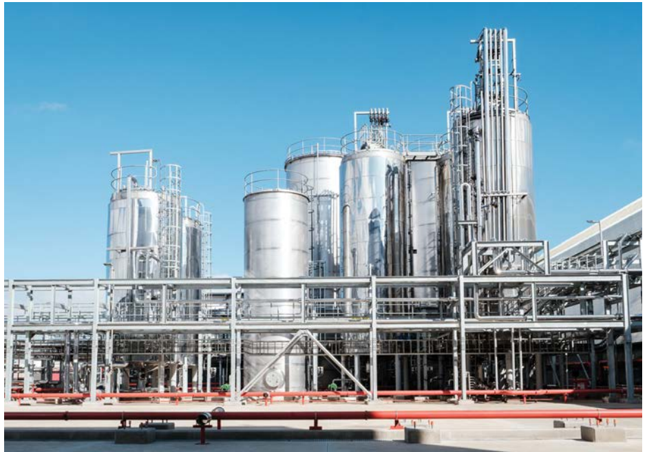
The new tank farm provides significantly expanded storage and blending capacity.
