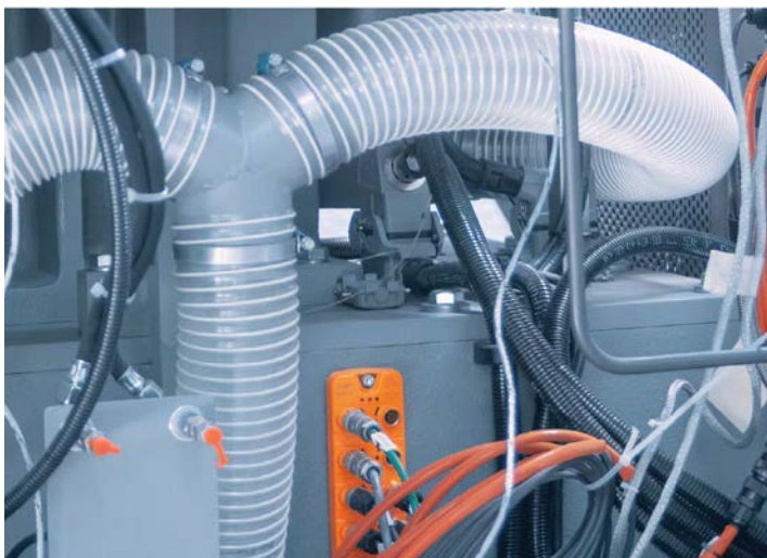
The sensor data from the recycling plant is collected decentrally via an IO-Link master and forwarded to the control system in bundled form.
