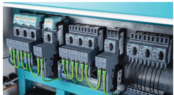
SIRIUS 3RC7 intelligent link modules in the cabinet.
