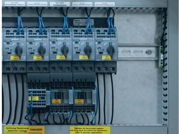
The evaluation electronics in the control cabinet process the data from the vibration sensors and transmit the results via Ethernet to the gateway, the IIoT controller from ifm.
