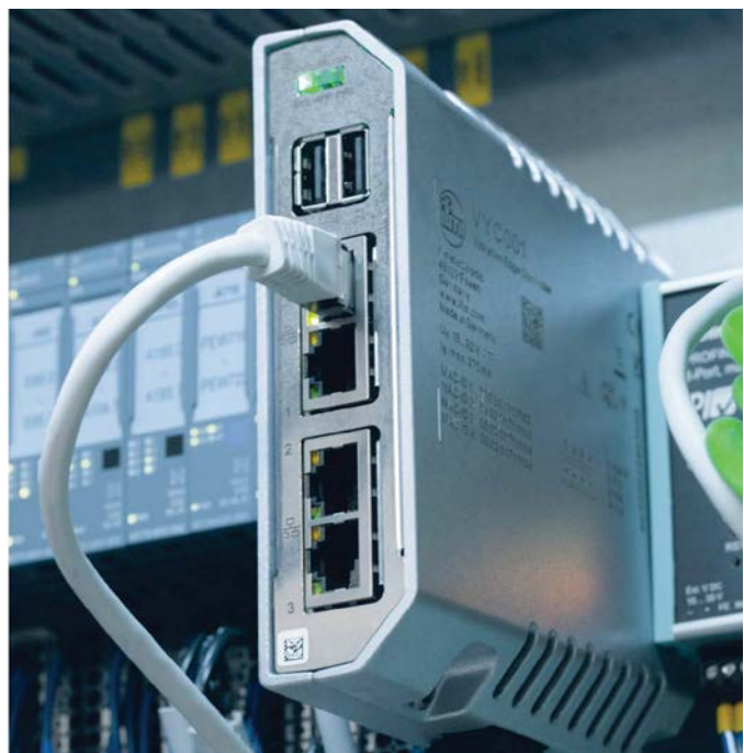
The IIoT controller transmits all sensor data to the higher IT level, where it can be accessed by EREMA customers at any time on a laptop or smartphone.
