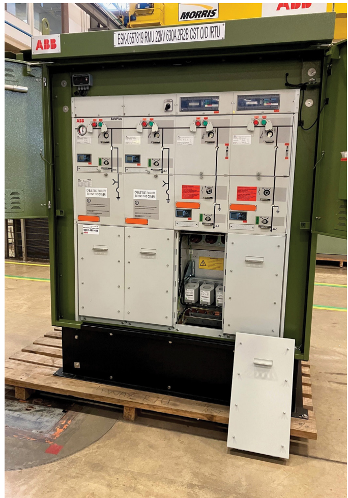
The Electrification Products division is playing a part in progressing ABB's regional production capabilities, with local manufacture of compact secondary substations, for example.
