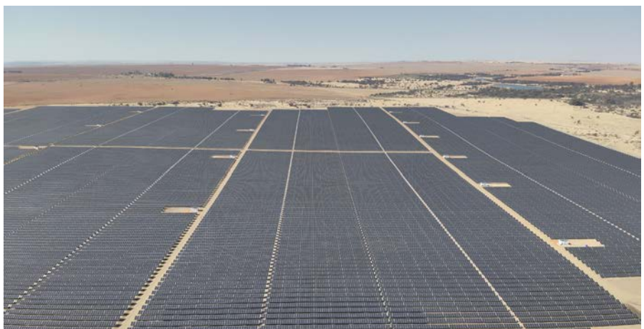
SOLA Group's Springbok Solar Power Plant, brought online ahead of schedule, is a pioneering multi-offtaker project supplying clean electricity to buyers nationwide.
