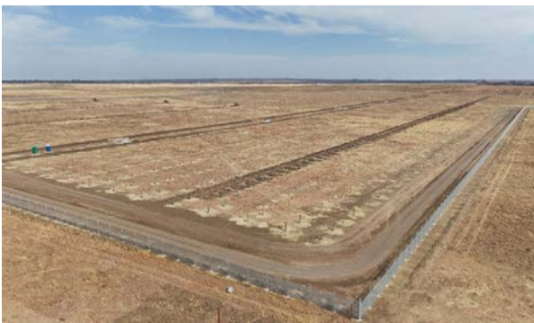
The 506 MW Khauta Cluster covers a 560-hectare site and will include a shared switching station and IPP substation.
