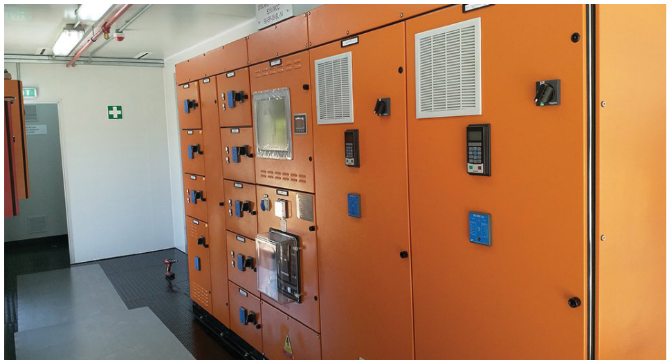
Today, Iritron assembles its electrical control panels and motor control centres in-house to ensure quality and on-time supply.
