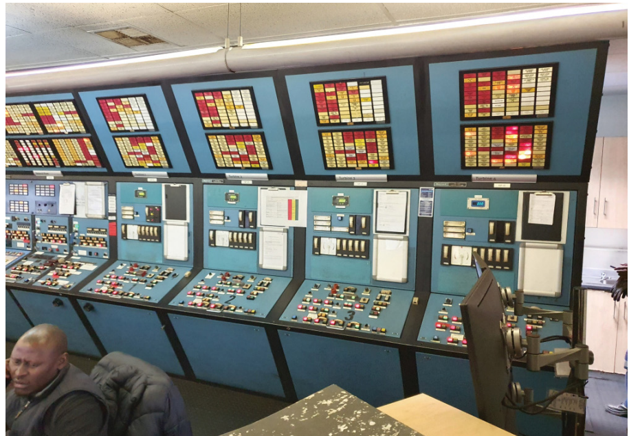
Maxiflex pole-mounted RTUs are interfaced to a central control room, to enable remote monitoring and resets when necessary.
