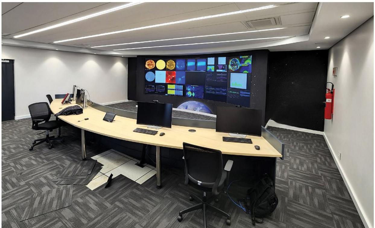
A smart control centre supplied and installed by Iritron.
