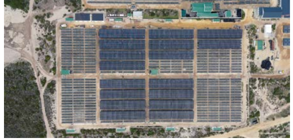
SPS has installed a solar PV plant with battery energy storage for leading abalone farming company Aqunion.
