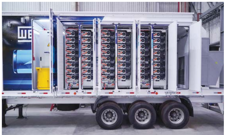
A BESS mobile solution (1 MW/1 MWh).
