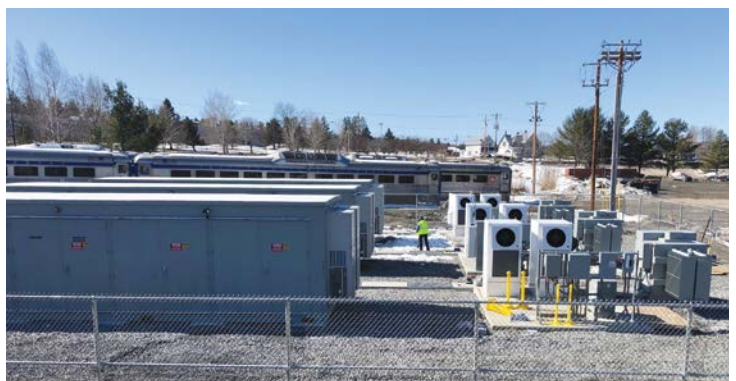
WEG BESS providing frequency regulation and ancillary services (5 MW/16 MWh).
