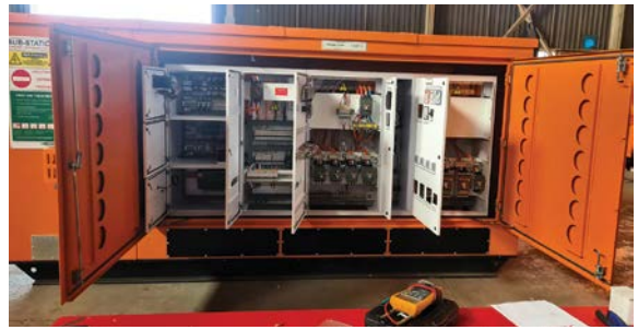
Each mini-substation is equipped with a control system that allows for the protection functions to be monitored remotely.
