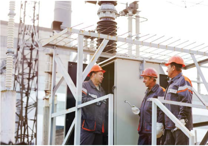
Electrical technicians who have the specialist knowledge required to monitor and diagnose faults in analogue systems are being called on to learn new skills as the digital grid takes form.
