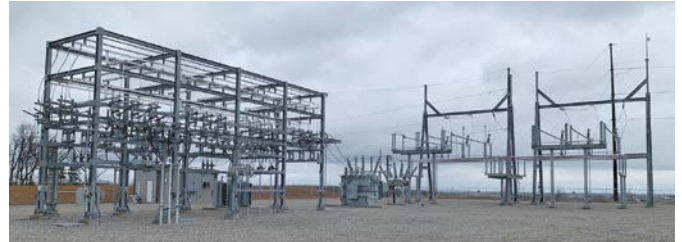
Some utilities are starting to move towards increased virtualisation in a digital substation model; most are still investigating the potential benefits.
