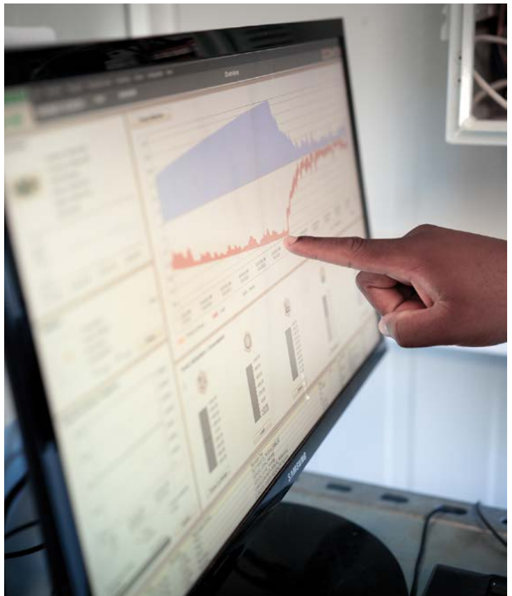
The microgrid incorporates a 75 kWp photovoltaic (PV) system, a diesel generator, and a battery storage system, all controlled by a Siemens SICAM Microgrid Controller.
