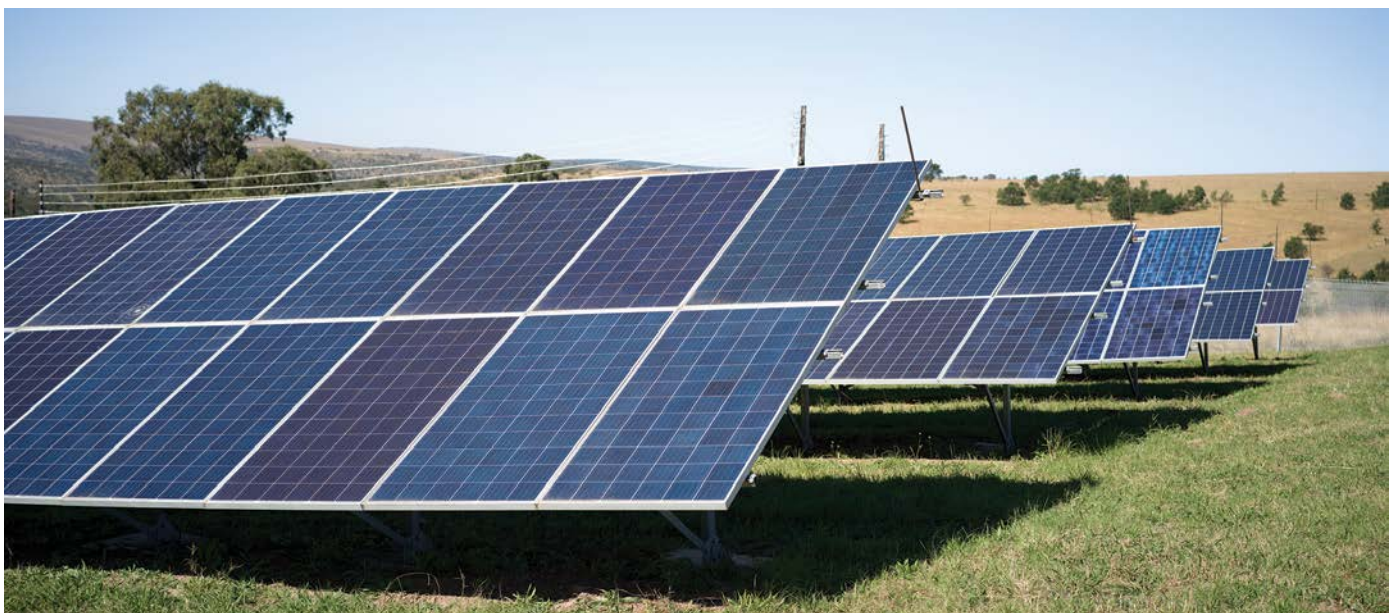
With the microgrid installed, Upper Blinkwater in the Eastern Cape, a small remote village never previously served by the national electricity supply grid, now has access to electricity.
