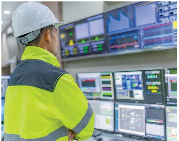
Using the MQTT networking platform and IIoT technologies, organisations can monitor plant and assets from anywhere.
