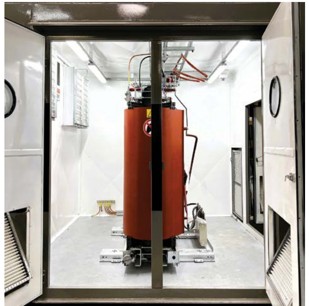
A dry-type transformer installed in a modular substation for a data centre.
