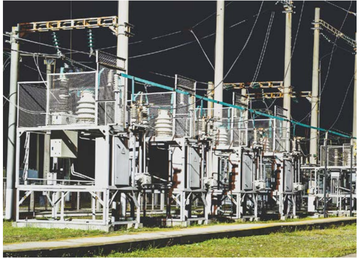
If aging substations are not well maintained, there is a higher risk of fire in transformers and other electrical equipment.
