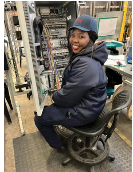
Wiring the switchgear is typically the most time-consuming aspect of production. (Photo: Electricity + Control)
