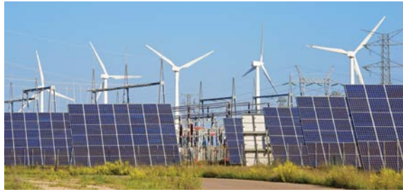
Hitachi Energy is a technology and solutions provider – meeting the needs of the changing energy system.
