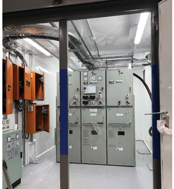
Modular substations, or E-houses, are prefabricated or modular structures that house electrical equipment and systems.
