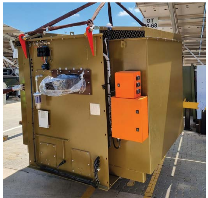
ArmCoil's MV substations, manufactured locally, offer versatility, reliability, safety and sustainability.
