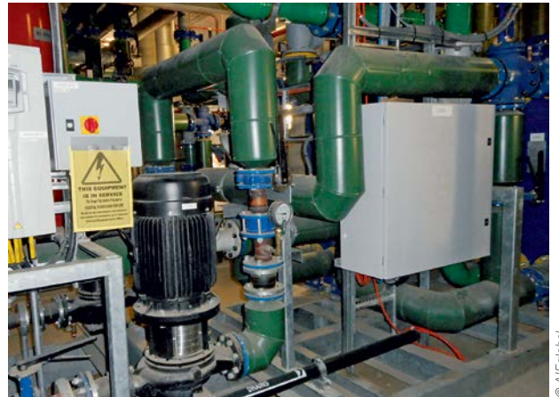
The EtherCAT I/Os installed on each genset significantly reduced the extent of cabling required to connect to the central control room.
