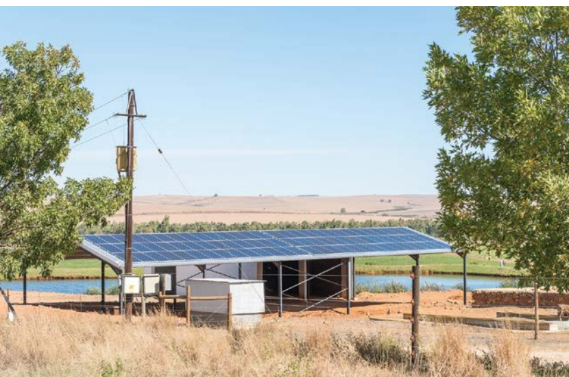
Localised microgrids can support energy sharing, energy savings and a stable supply for small communities.
