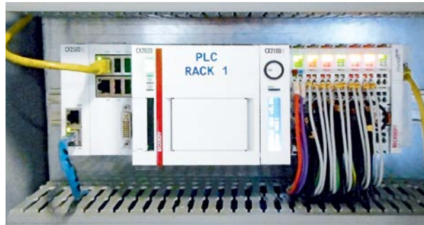
Seven CX2020 Embedded PCs were selected to automate the four 2 MW gensets, the heat exchangers and the overall plant control system, as well as the connection to the SCADA system.
