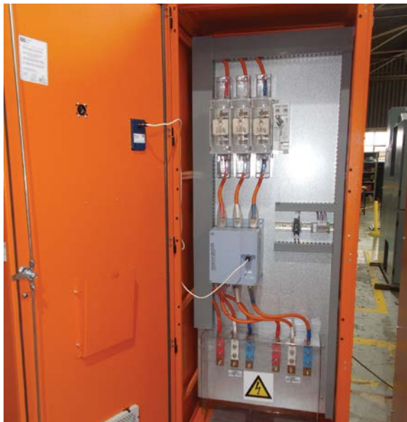
The standalone soft starter (185 kW/550 VAC) housed in an IP42 enclosure was designed for the tailings pumping motor control centre.
