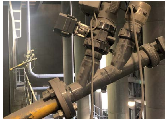
The Inspecta Automatic Purge System in application.
