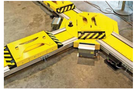
At the stoppers and other function modules, the eCart system communicates with the carts via NFC.
