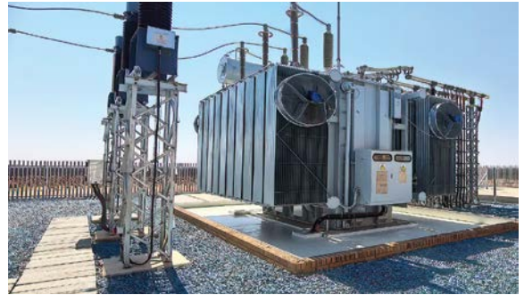
An ACTOM Power Transformers 40 MVA Class 1 power distribution transformer in a substation.
