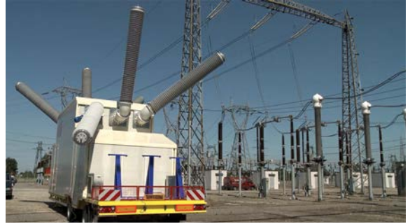
Modular mobile substations provide a rapid-response solution for major grid disruptions.
