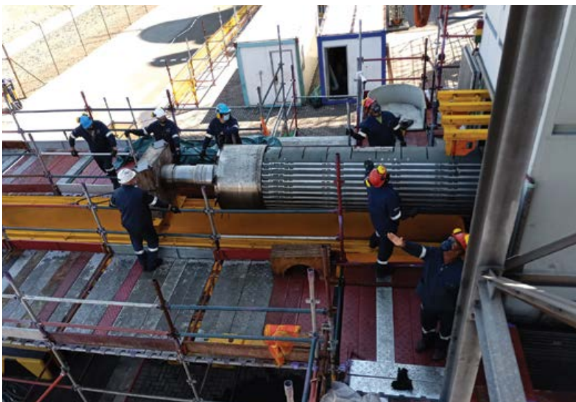
Members of the ACTOM Turbo Machines team at work on removing the 147 MVA rotor from the stator.
