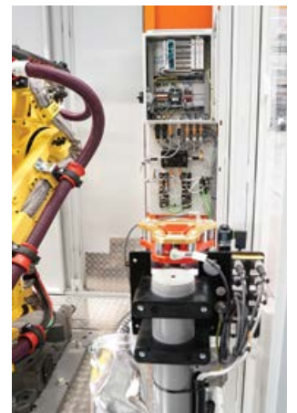
A decentralized safety solution installed.
