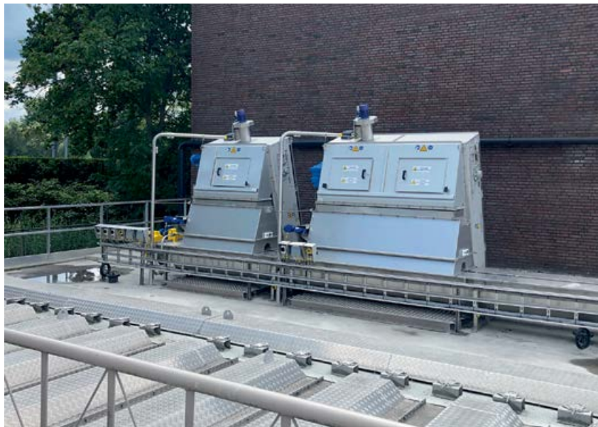
Sludge, sand, wood – the residual materials from wastewater treatment plants demand a lot from the deployed sensors.
