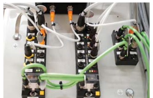
This safety application is controlled by the TBP (left) for testing in the factory. A Profisafe controller takes over the application in live operation at the plant. All actuators connected to the IO-Link master (centre) are safely disconnected by the TBSB Box (top).
