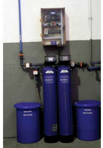
With the new PLC and software, Allmech's demin plants are more easily customisable and can include plant monitoring functionalities.
