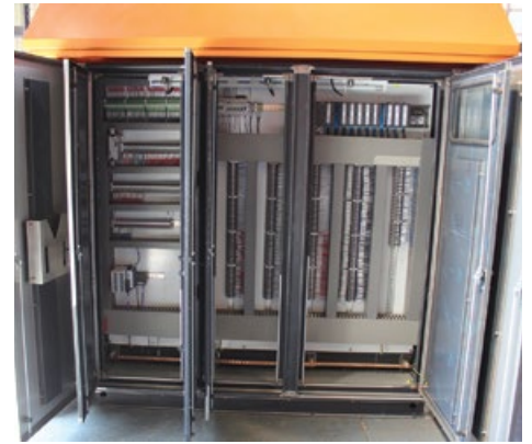
JB Switchgear is working on electrical panels, field junction boxes and other equipment at Sishen's Koketso project.
