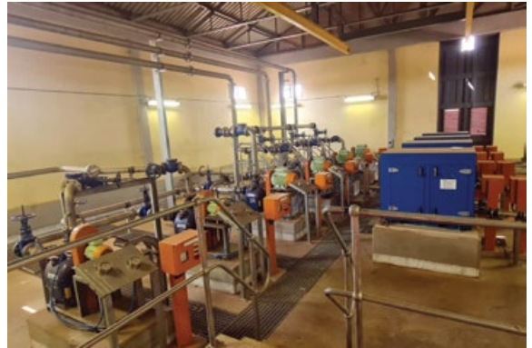
WEG motors in a de-gritting pump station.
