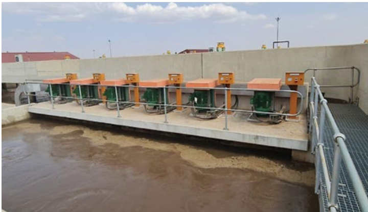
A water recycling installation driven by WEG motors.
