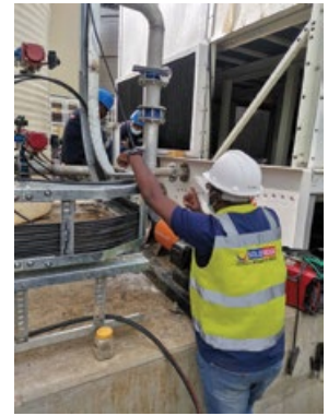
Solid Wedge team members on site, installing electrical & instrumentation systems at the new gold plant.
