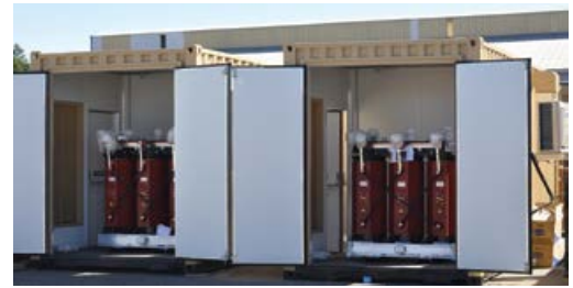
Custom-designed and -manufactured cast resin transformers in a specialised IP55 enclosure installed outdoors in a mining application.
