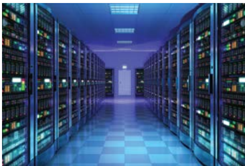
Colo facilities offer the advantage of specialist in-house expertise, which few enterprises will have in their own data centres.
