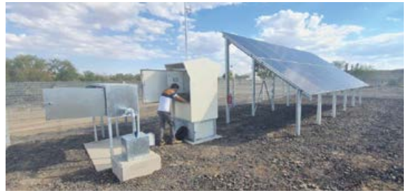
A modern telemetry and control system enables more efficient real-time management of scarce water resources.
