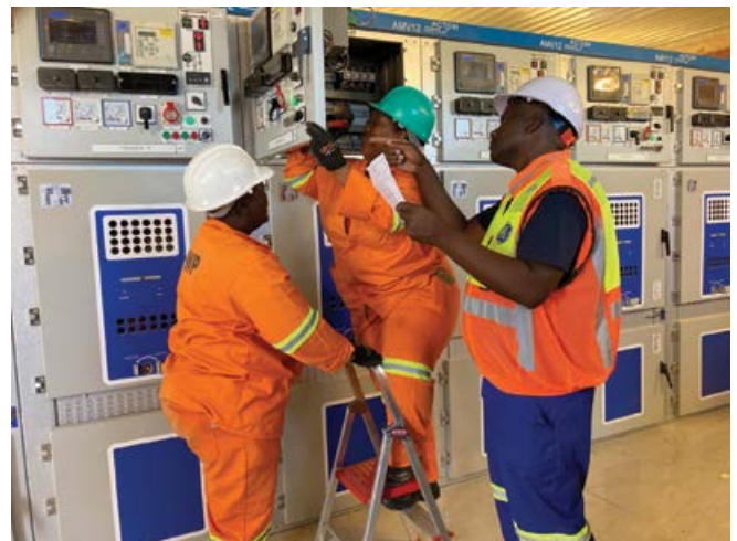
EPWP candidates assist with a wiring alteration on an AMV12 switchboard control cubicle, under the supervision of Kaizer Sithole from ACTOM Power Systems.
