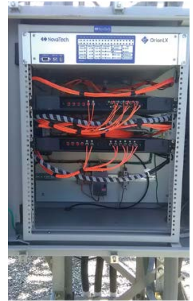
An OrionLX RTU cabinet installed at one of the substations.
