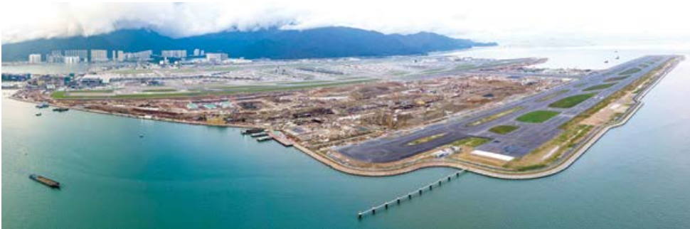
The third runway expansion at HKIA is one of the biggest airport construction projects currently under way.
