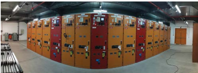
The project includes electrical motor control centres as well as other systems and equipment.
