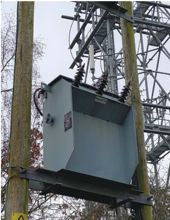
One of the transformers feeding power to the borehole pump system at an EA groundwater site.
