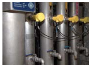
Pressure measurement with VEGABAR 82 in the cleaning system.
