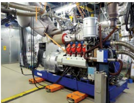
Rolls-Royce has commissioned its first in-house test stand for mtu hydrogen engines at its Augsburg site.
