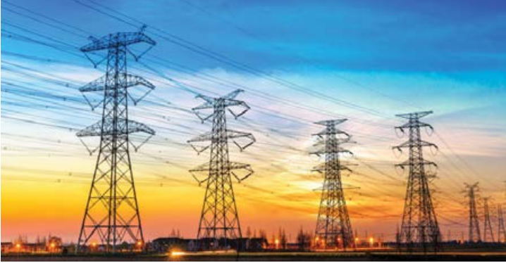
A critical enabler for the large scale and rapid pace of renewables deployment is the modernisation, expansion and strengthening of the national power grid.
