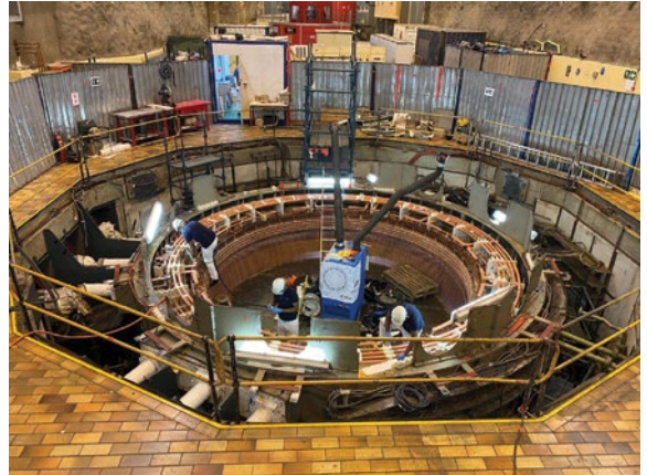
After the rotor was removed, M&C technicians set to work inside the stator to install several hundred stator bars as part of the stator winding contract.
