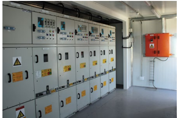
Switchgear installed inside one of the six-metre containerised substations.
