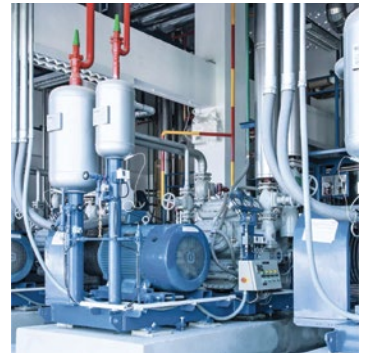
Consistent monitoring of compressors allows for maintenance to be carried out as needed, saving time and costs.
