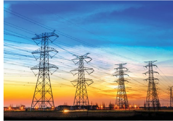
Eskom's planned investment in the national transmission grid amounts to R178 billion over the next 10 years.
