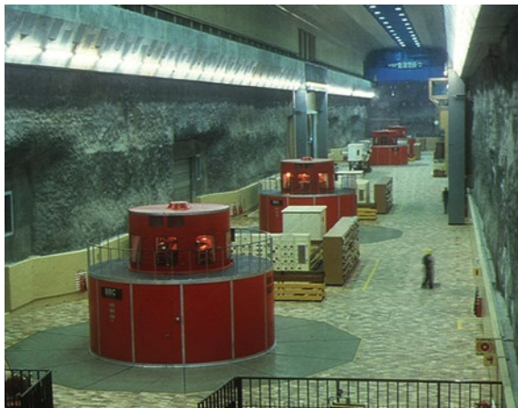
The turbine hall at Eskom's Drakensberg pumped storage power station.
