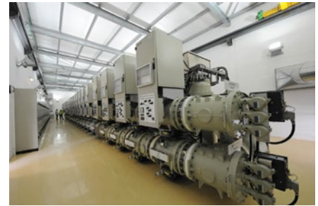
Gas-insulated switchgear in the City of Cape Town's 132 kV Foreshore indoor substation, where ACTOM Power Systems supplied and installed the electrical works in 2009.
