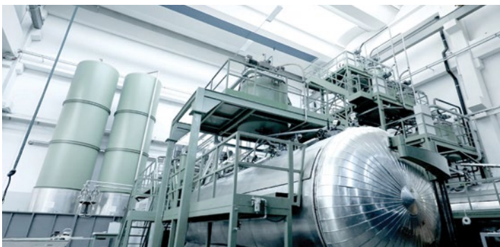
A casting plant with specialised resin mixing facility, unique to cast resin transformers.
