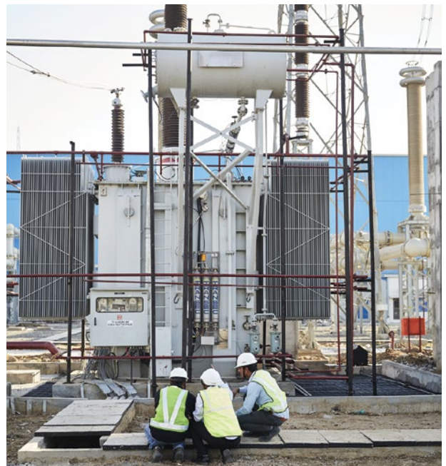
Transformer performance and quality have a major impact on the availability of power generated and the reliability of the network.
