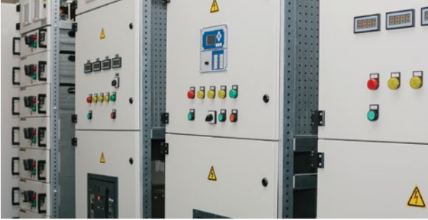
Surge voltages can damage electronic components and pose a risk to plant availability.
