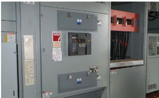
The bottled water company installed 24-inch IR windows in main breaker bus cabinets.
