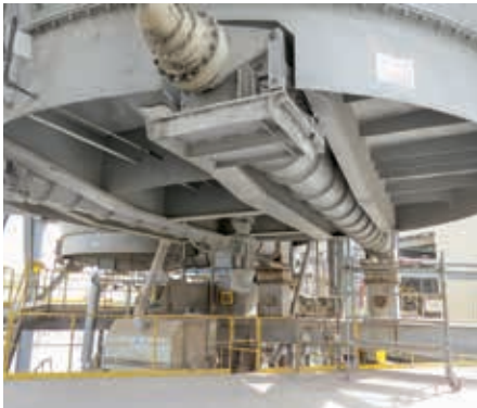
A large agitator with sharp knives ploughs its way through the mass of waste materials in the storage silo.
