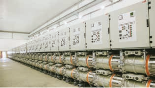
Gas-insulated switchgear at Johannesburg's Sebenza substation.
