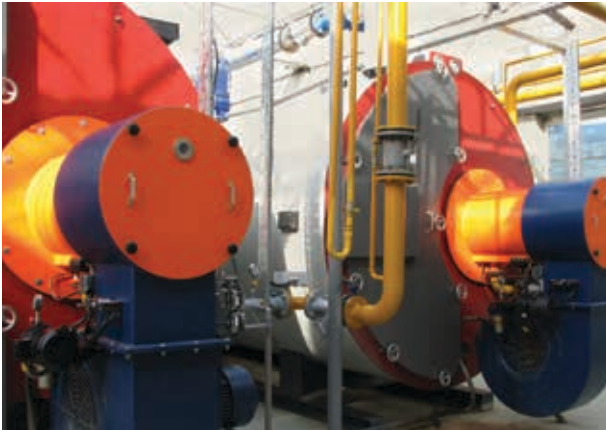
Industrial steam boilers used in process plants also require regular checks and testing to maintain optimum operating efficiency.
