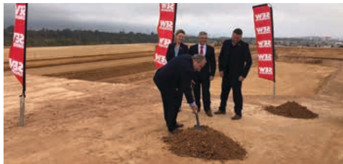
SEW-Eurodrive MD, Raymond Obermeyer and colleagues breaking ground on the site of the new facilities.
