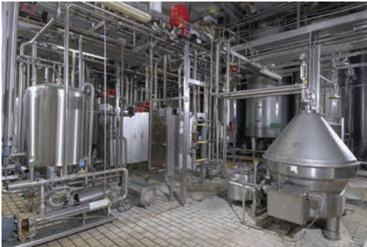
Process automation technology provides customers with optimal routing and 'cleaning in place'.
