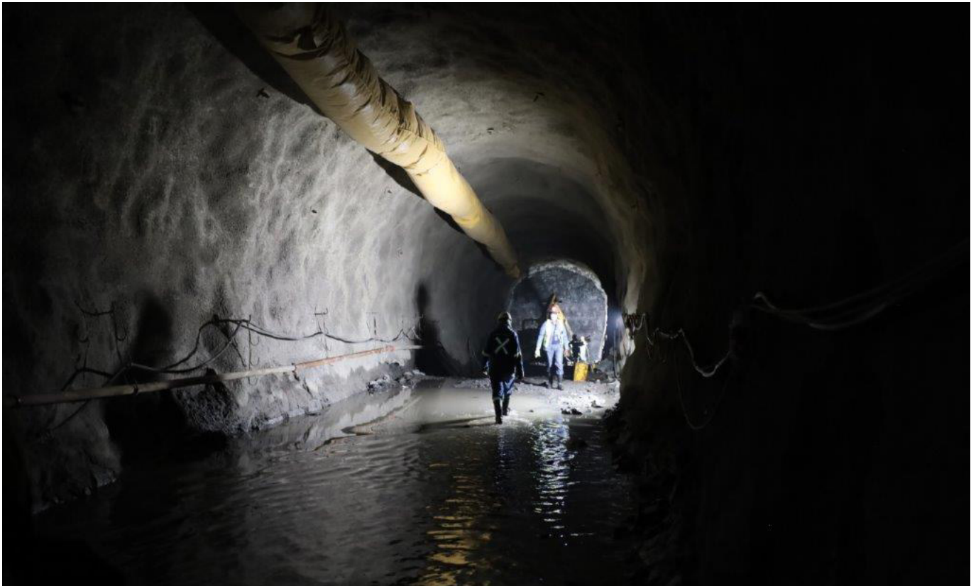
The Polihali Transfer Tunnel is one of the most technically demanding components of the Lesotho Highlands Water Project Phase II.
