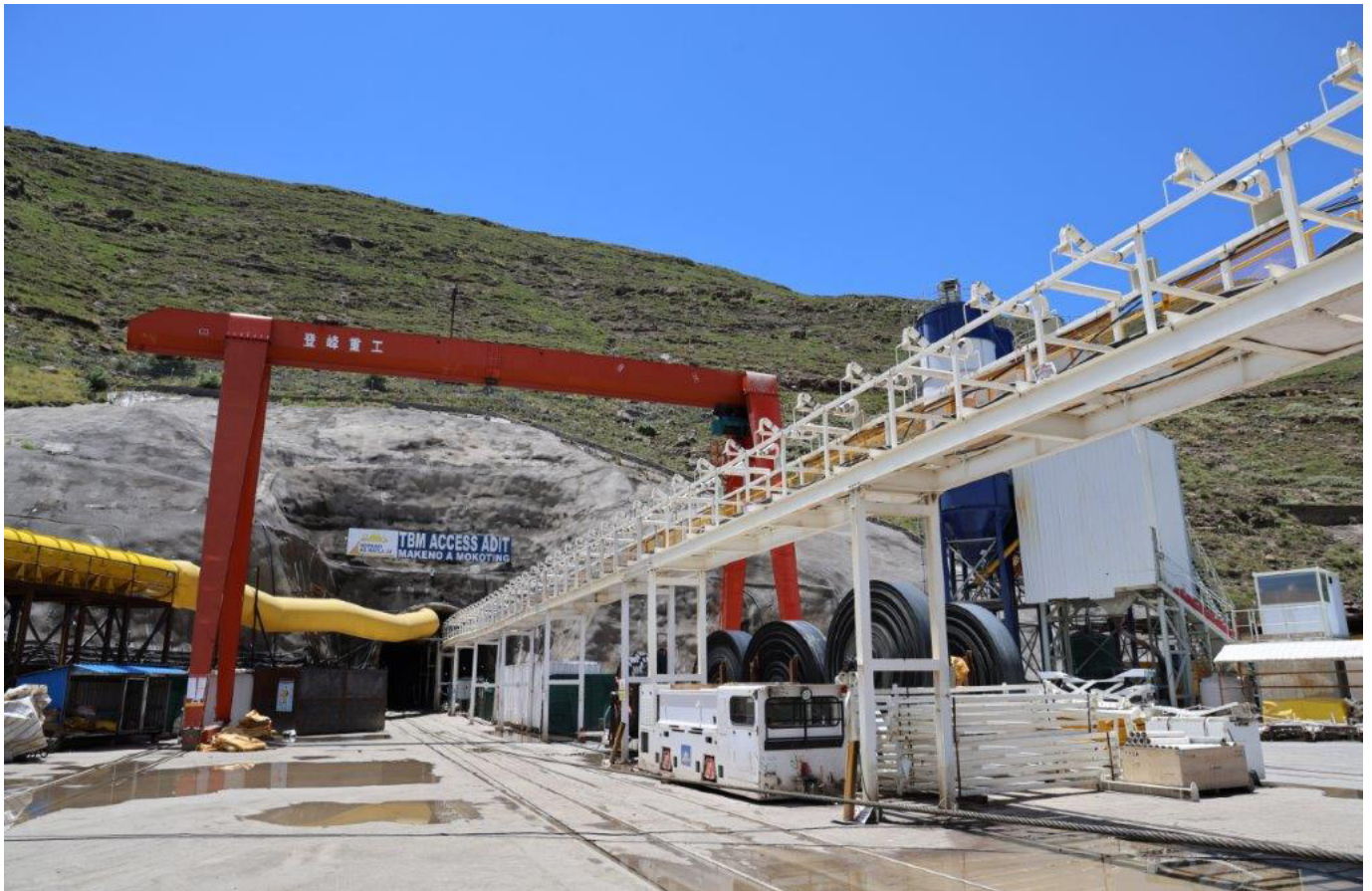
Polihali Dam incorporates a 5 m-diameter TBM tunnel with intake works, gate shaft, and outlet connecting to Katse Reservoir.
