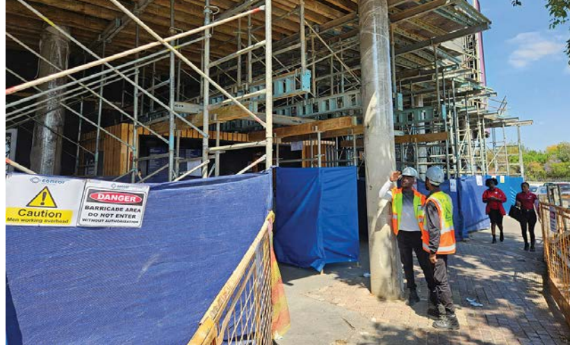
Concor's safety personnel carry out detailed inspections of formwork and public-interface zones to ensure secure structures and safe access around active construction areas.
