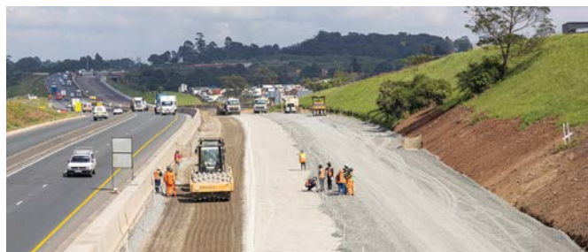
From national highways to municipal and rural access roads, AfriSam Roadstab Cement continues to underpin critical transport infrastructure across Southern Africa.
