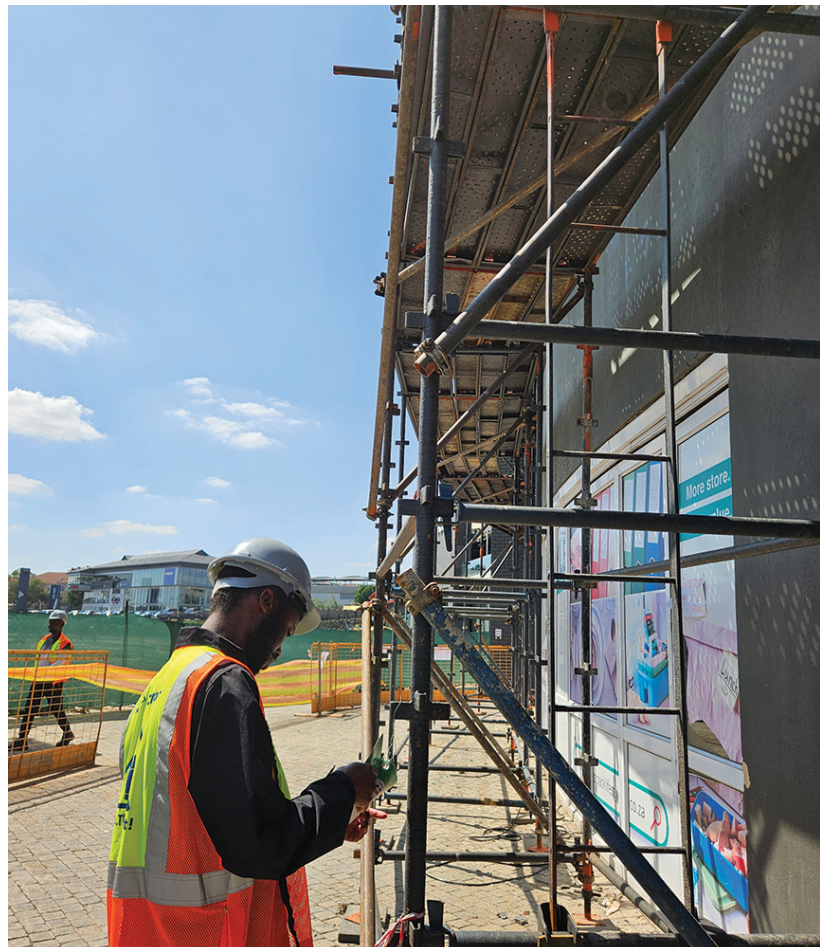
A routine scaffold inspection is undertaken to confirm structural stability and compliance, reinforcing Concor's focus on preventing fall-related incidents on site.
