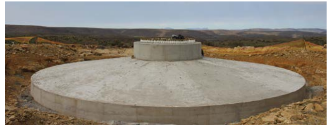
From turbine foundations to working platforms and access roads, each element showcases the technical expertise of civil engineering contractors.
