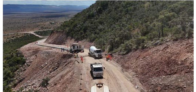
Access and haul routes enable the transport, installation and ongoing servicing of major renewable energy components in hard-to-reach areas.
