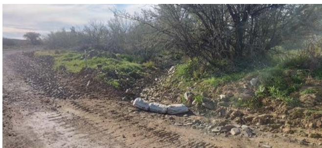
A sandbag silt trap is installed at the watercourse crossing on the Karreebosch Wind Farm facility to safeguard the environment during construction.
