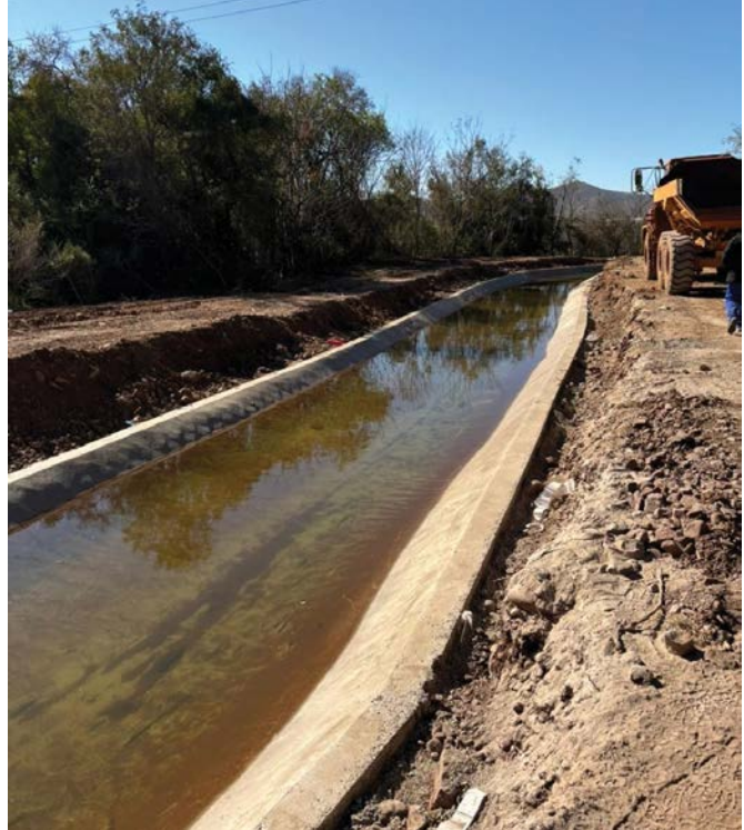
Fibertex Nonwovens SA has recently collaborated with a leading construction company - through the supply of an eco-friendly geosynthetic solution, designed to combat soil erosion at a new solar power plant in South Africa.
