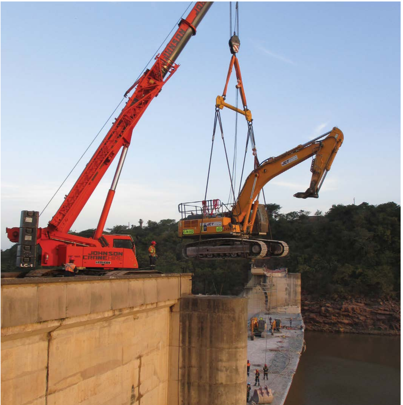
Jet Demolition used cranes to lower the demolition excavator onto the Hazelmere dam wall.
