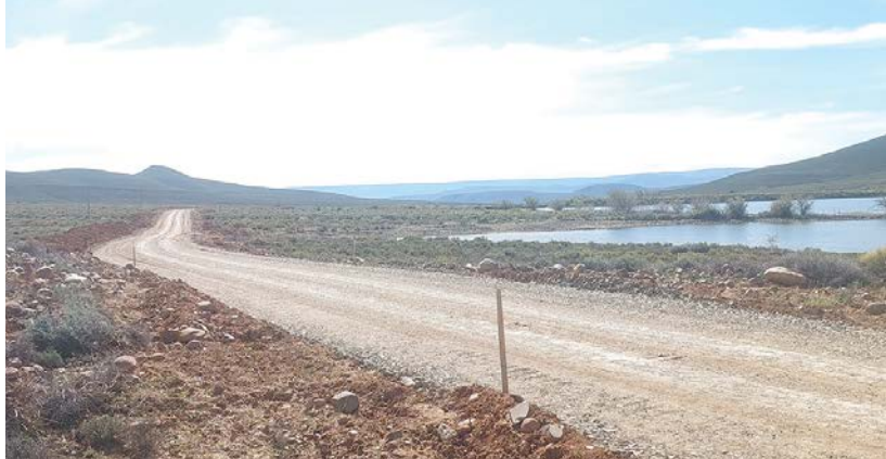
At the Karreebosch Wind Farm facility, Concor ensures careful management of the road servitude close to the water body.
