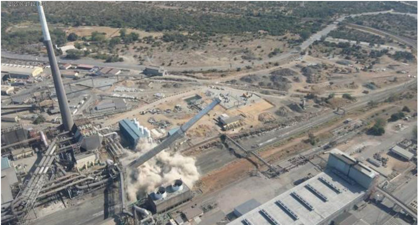
Palabora Mining Company (PMC) - Compromised Converter Stack.
