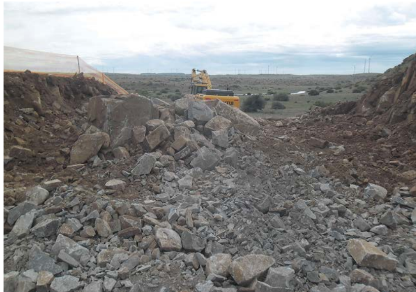
Cut-to-fill activities in progress on the De Aar 2 South Wind Energy Facility project, optimising on-site material use for road construction and turbine platform preparation.
