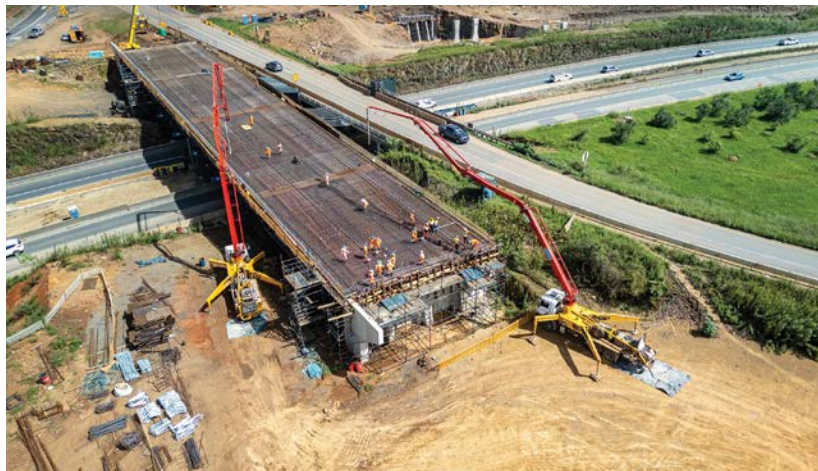
The critical aspect of the project was to avoid disrupting traffic on the N3 as well as over the existing Market Road bridge close to the N3.
