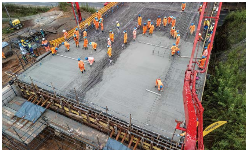
Due to the dense steel reinforcement, maintaining a concrete slump consistent within the specification was essential.
