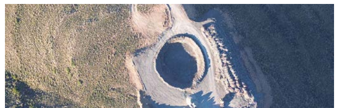
A close-up view captures the excavation of a wind turbine base underway at Karreebosch Wind Farm, where Concor is preparing the foundation to exact specifications based on detailed geotechnical investigations.
