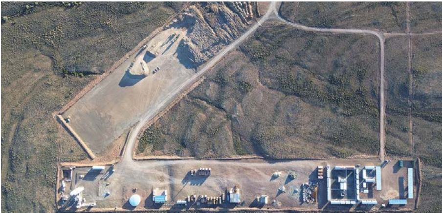
Early project works undertaken by Concor include establishing access roads, site offices and an on-site batching plant, in preparation for the large volumes of concrete needed for the turbine foundations.
