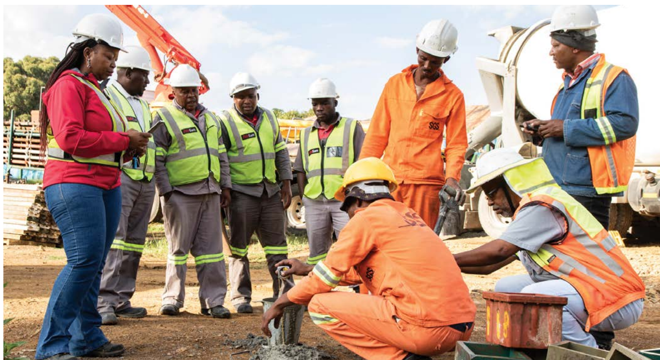
A key focus for AfriSam is developing and retaining the skills the construction sector demands.
