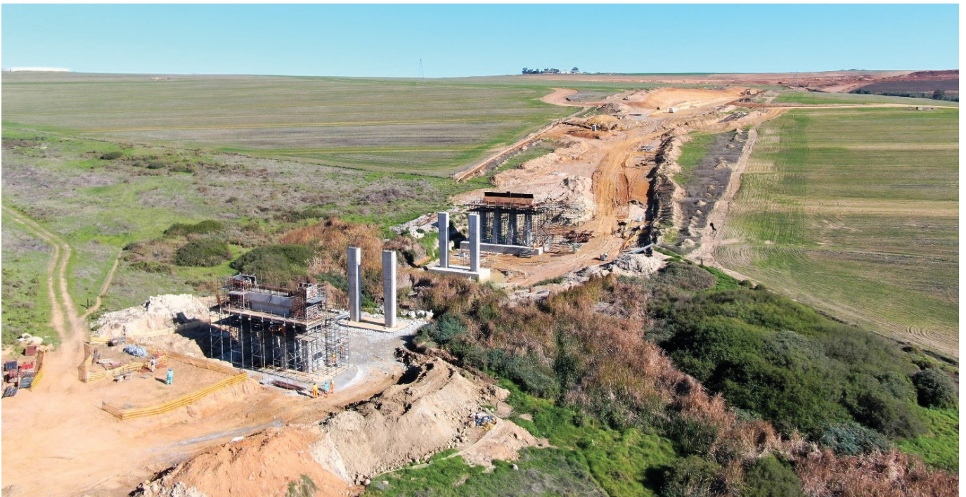
The Malmesbury Bypass is a critical infrastructure project for the Western Cape.
