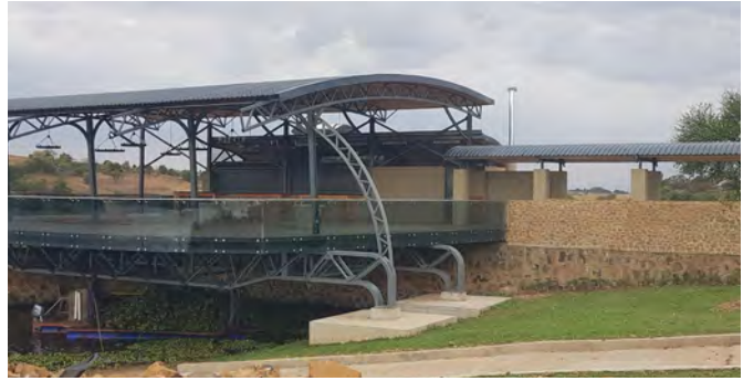
EB construction could rely on the quality of AfriSam's readymix concrete for the construction of a complex structure over a dam.
