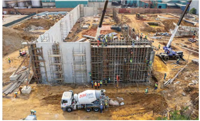
The project includes a large 30 m by 90 m bunker with 11.5 m high walls, topped with a 5 m steel structure.
