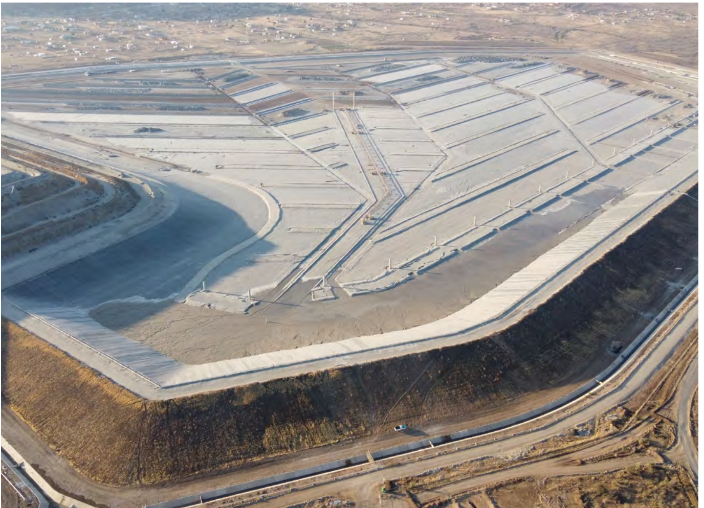
SRK is involved in various large tailings dams, including the construction of new dams and the strengthening of existing dams.
