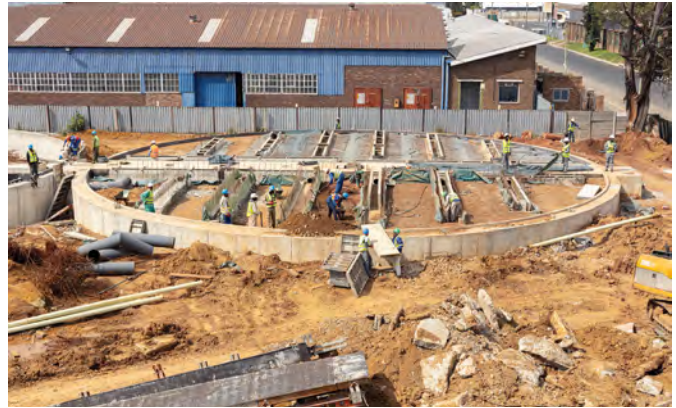
The concrete work also included the bases for four silos, using a total of 700 m 3 of concrete.
