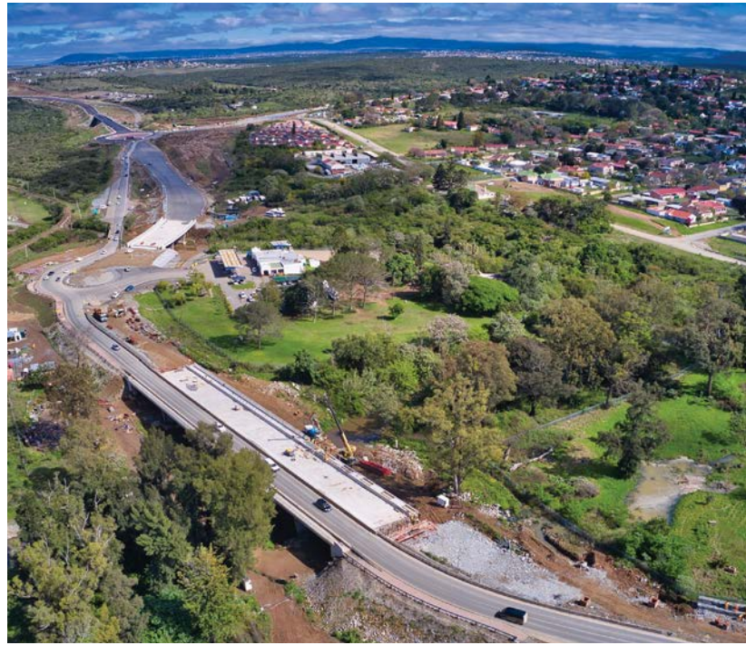
The Tshoxa 1 Bridge reflects the successful integration of concrete's functionality and aesthetics to enhance the quality of life through infrastructure development.
