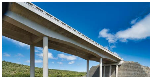
The Tshoxa 1 Bridge project made a significant impact on the local community by directing 30% of its contract spend to local subcontractors and suppliers.
