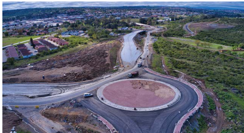
The concrete mix design addressed challenges posed by the region's natural sand quality by replacing it with carefully selected quarry dust.
