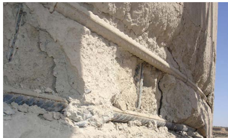
Appropriate concrete design and construction including adequate measures to prevent concrete corrosion, will save asset owners significantly in major repairs further down the line.
