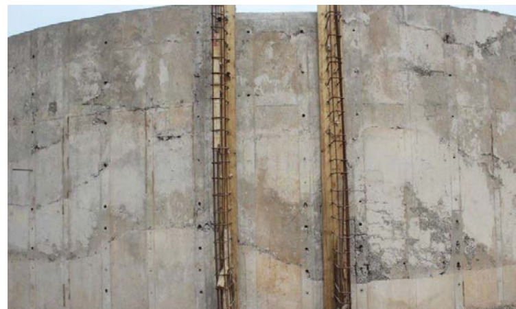
Appearing as cracks, honeycombing and areas with exposed aggregate and reinforcing, cold-joint lifts prevent a strong, water-tight bond between the layers in the reservoir wall.
