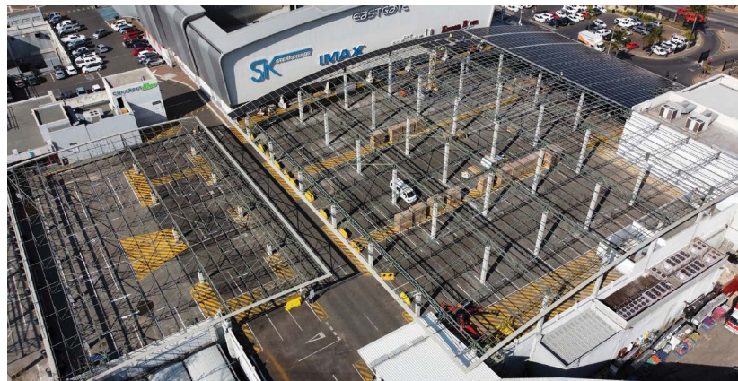
An aerial view showing the steel framework with some of the solar panels already installed.
