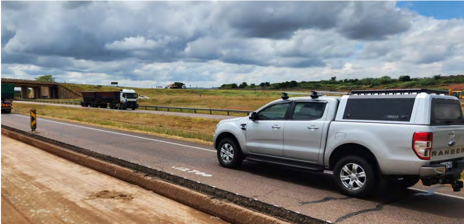
G4 Civils started with the construction work on the project in January 2022 and is expected to complete the work scope in August 2023.
