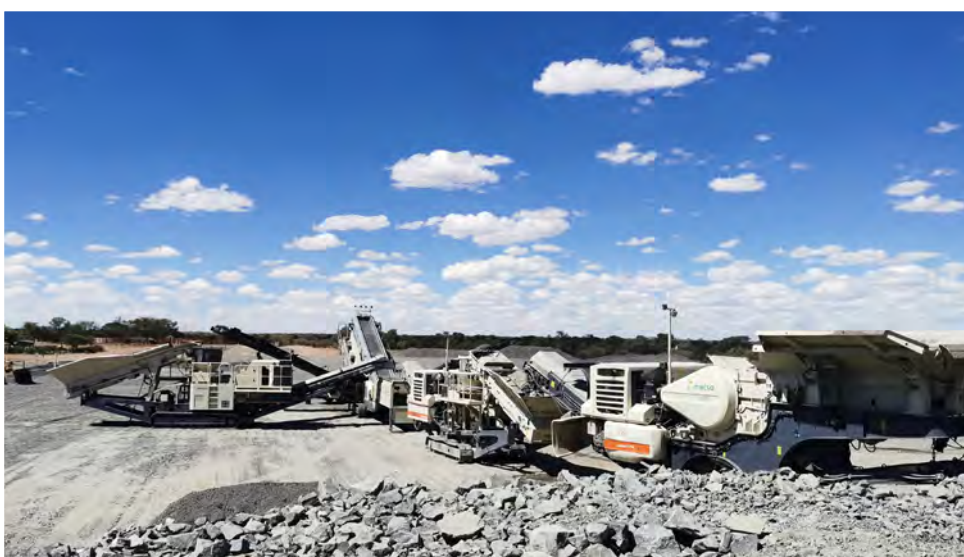
A Lokotrack mobile train for aggregates in road construction working in Namibia.
