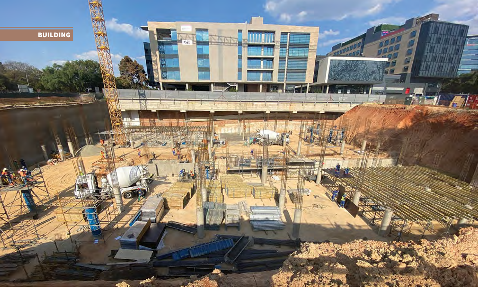
Construction of the four storey, three and a half basement building began in March 2021 with handover in February 2022.
