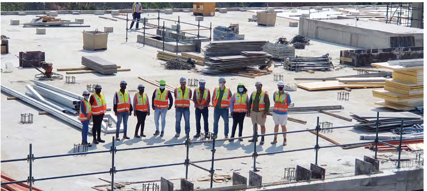
The Concor team for the Ikusasa project on the topped out structure.
