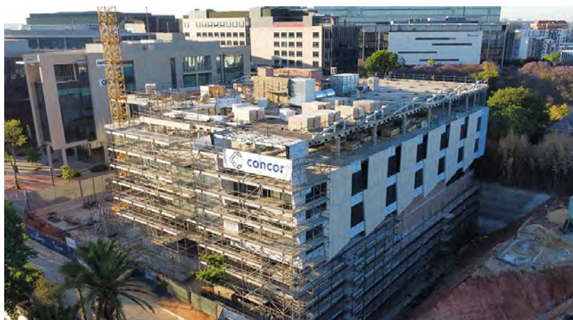
As a fast track project, success was achieved on the Ikusasa project through tight control over scheduling, and by prioritising sustainability and zero harm principles.
