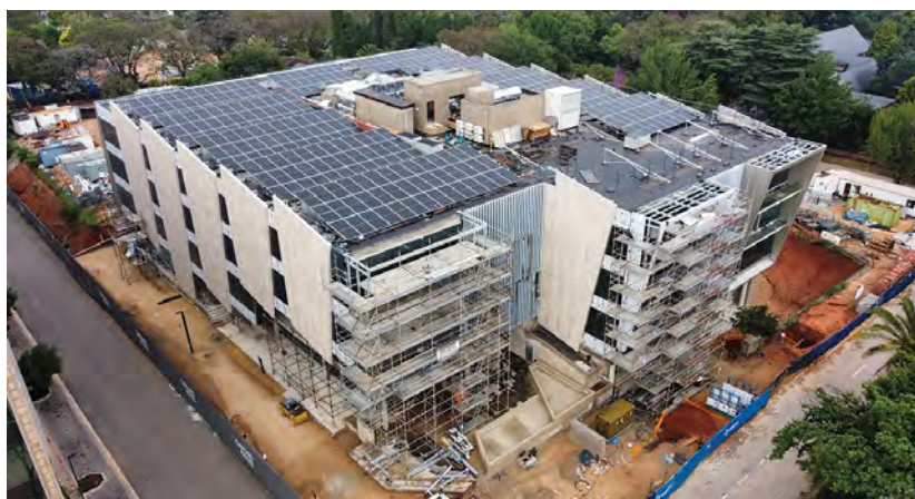
Ikusasa’s Green Star SA Net Zero Carbon Level 1 means that the building generates as much energy on site as the base building requires. This includes the use of a photovoltaic solar generation system on the roof.
