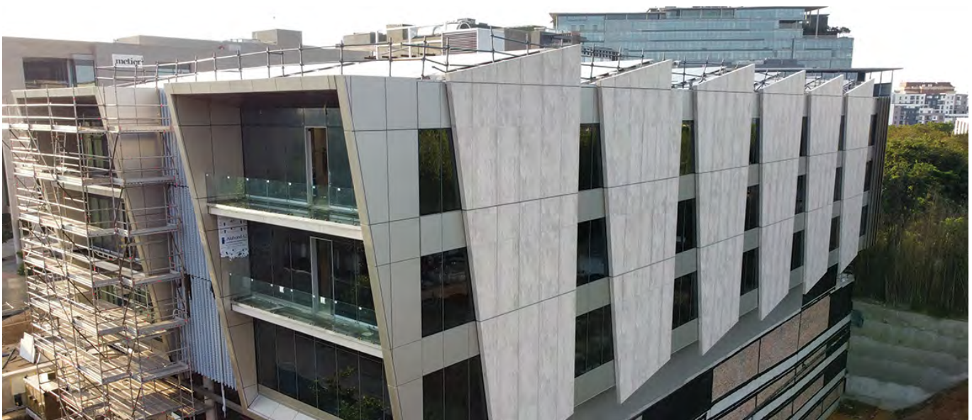
Accurate dimensioning of the façade was possible using sophisticated software that could model the full façade around the concrete structure. These approaches meant Concor unlocked two long lead materials: the glass and façade tiling.
