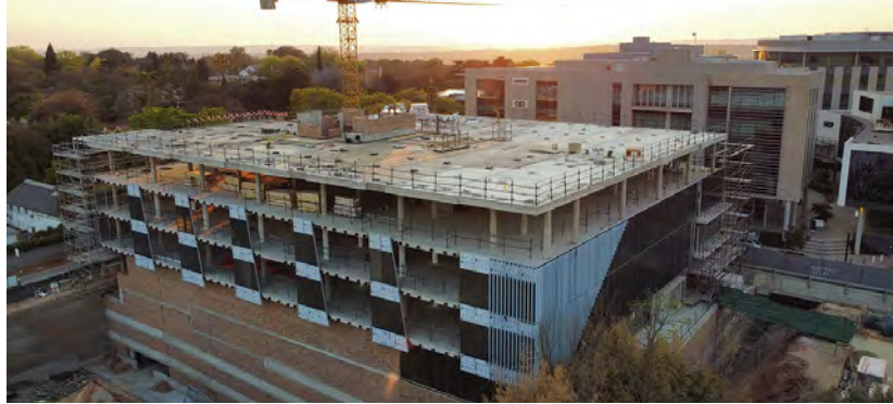
Installation of the façade starting; this unitised system was less labour intensive to install and did not require a full façade scaffold for installation. This also reduced cost and time.
