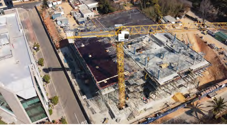
The concrete structure on the Ikusasa project progressing with the third floor construction underway.
