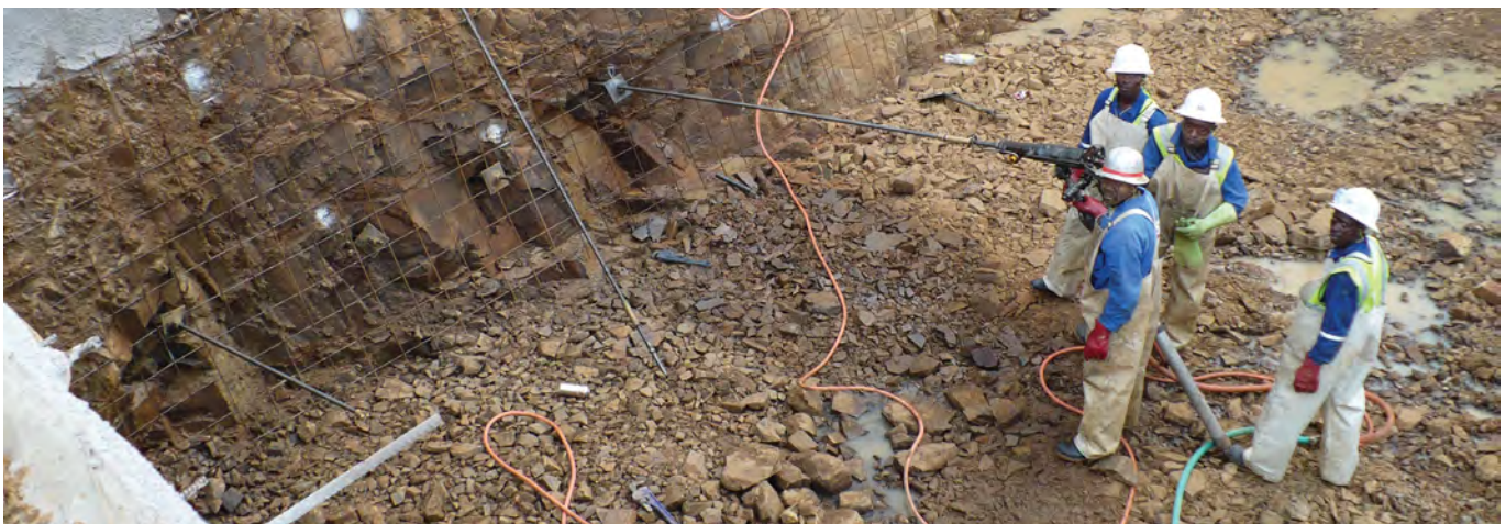
Not only must engineering structures be technically sound, cost-effective and safe, they must also be environmentally and socially responsible.
