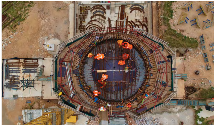
A bird's eye view of the steel fixing on the bifurcation lift soffit slab.
