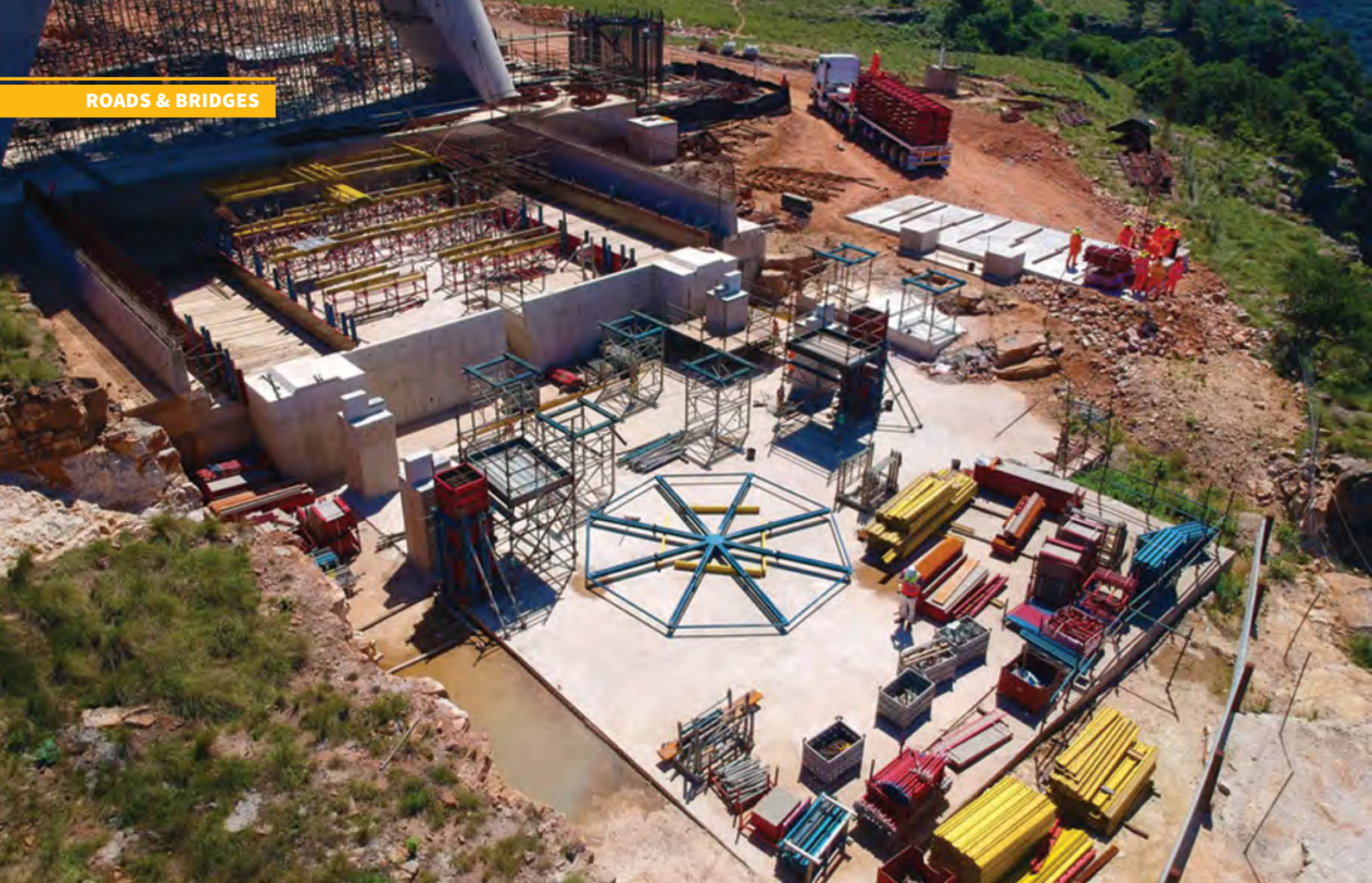
The South area preparing for the arrival of the deck segment in November 2022.
