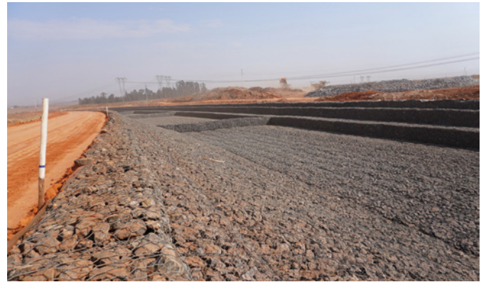
Construction of the stream saw over 4 100 gabion baskets and some 42 000 t of rock being used.
