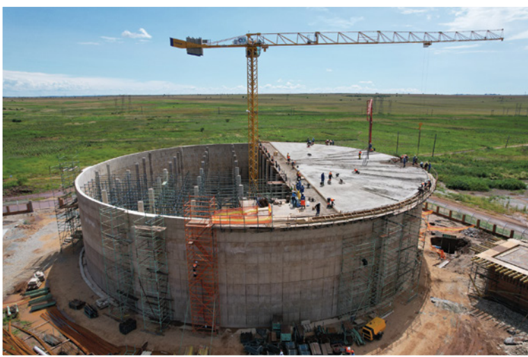
The Khutsong reservoir is Africa's first round prestressed raft floor to deal with dolomitic ground conditions.
