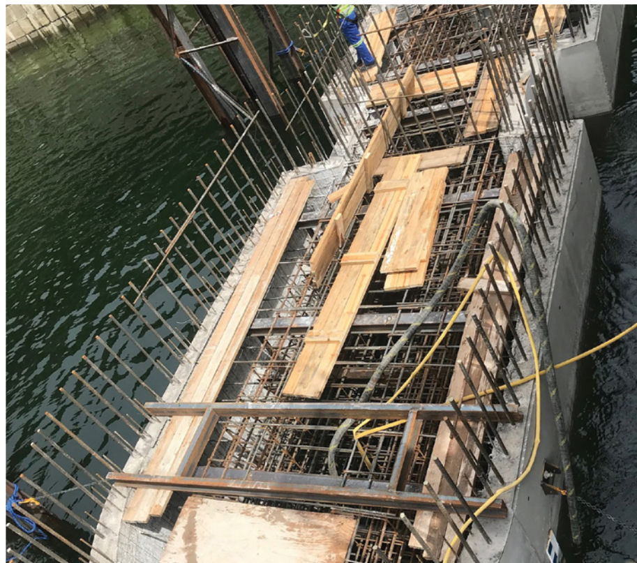
Construction of one of the seven Kariba Dam pier bases to be submerged under water.
