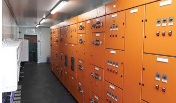
A containerised motor control centre built by Hamar Controls for a mine in Tanzania.
