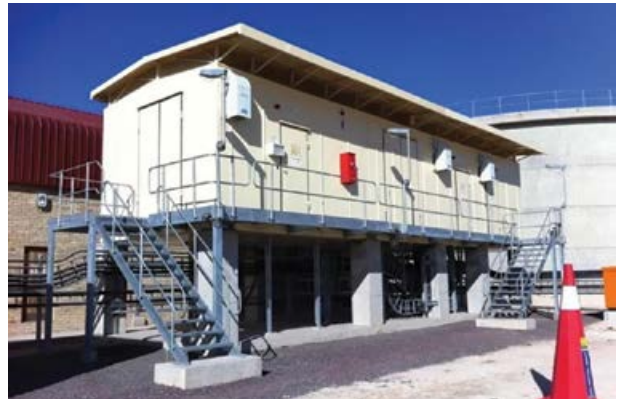
JB Switchgear also supplies prefabricated modular substations, or E-houses, built to clients' specifications, a cost-effective alternative to conventional brick and mortar buildings.
