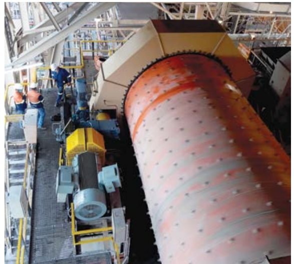
The first girth gear was installed on one of Venetia's secondary scrubbers last year.
