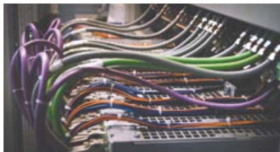
Together with HMIs, PLCs, which store and execute logical sequencing processes, are fundamental to automation and control systems.
