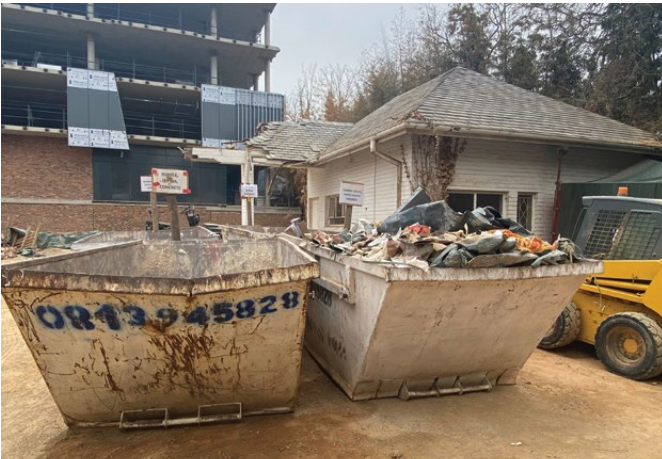
Left: It is important to carefully manage waste on site, ensuring each category remains uncontaminated. Right: It is important that waste is uncontaminated, and this requires ongoing training of subcontractors.
