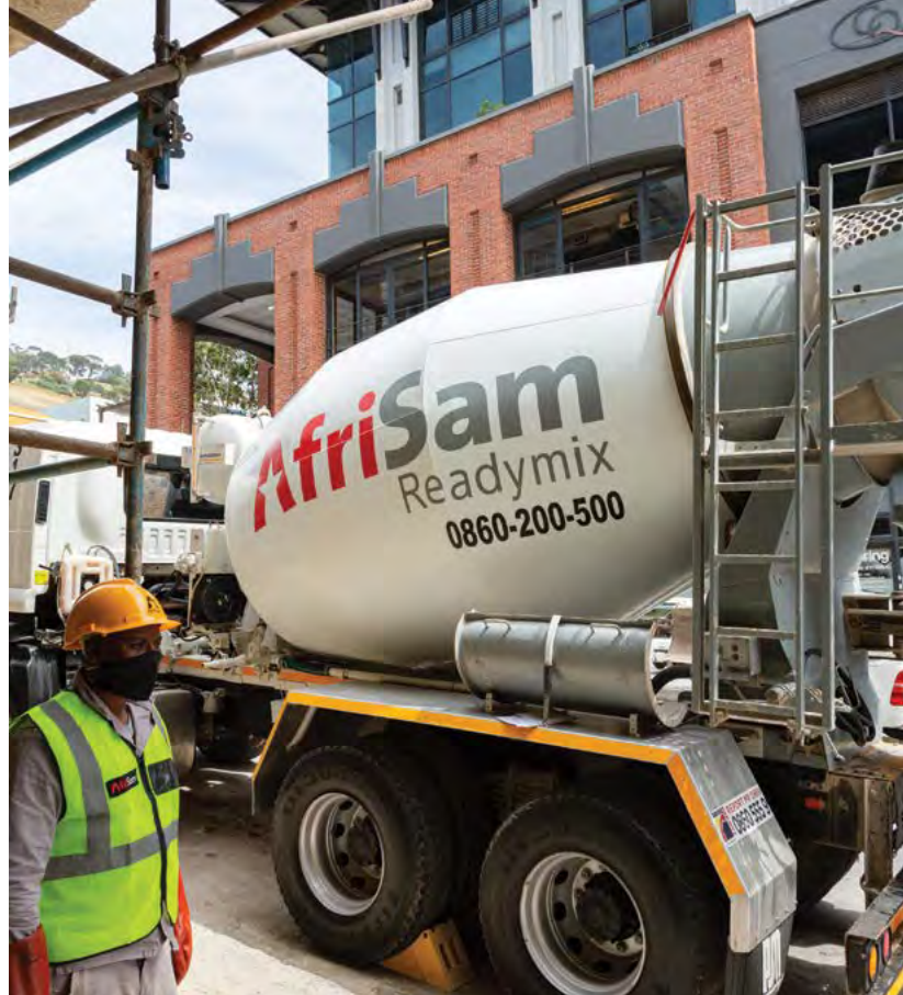
AfriSam supplied 9 700 m 3 of concrete for this project, mostly from its Woodstock plant.
