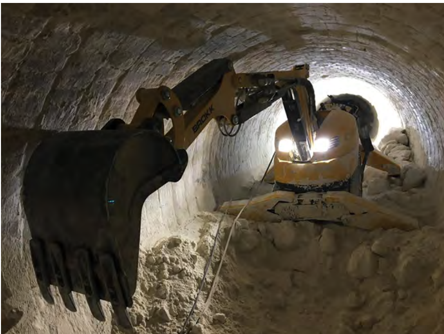
Demolition robots can be paired with a bucket to increase efficiency for a number of confined applications such as excavation, digging trenches, material handling, sorting, separating and loading debris.
