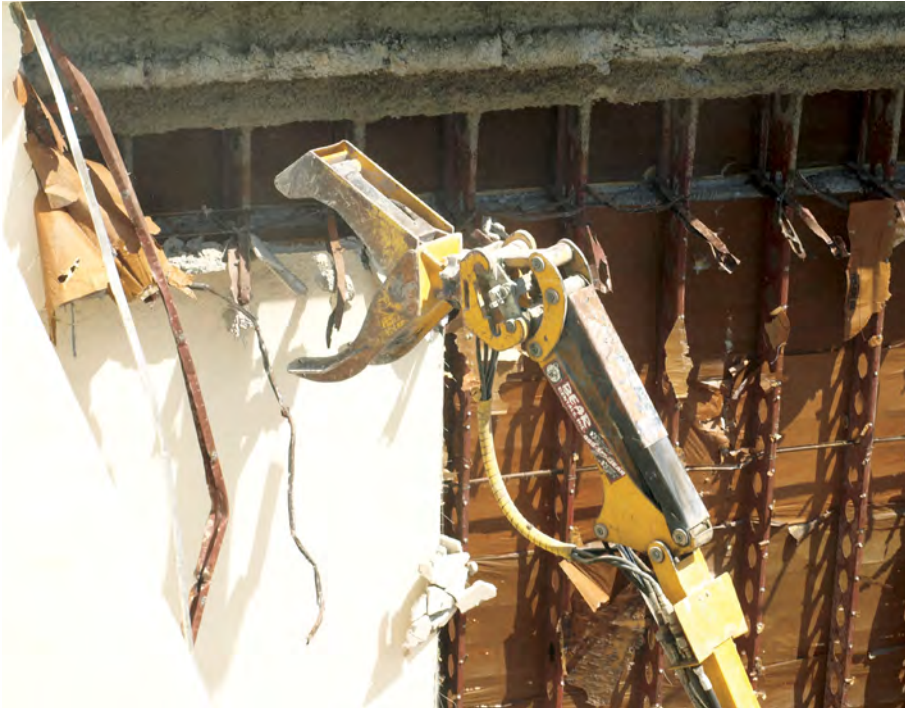
When paired with a flexible remote-controlled machine, the grapple can easily grasp and pull down structural elements.
