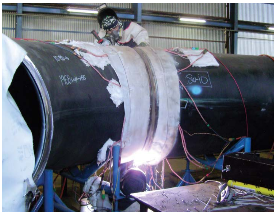
Aurex Constructors’ Chamdor facility has maintained ISO 3834-2 since 2012, ensuring consistent welding quality and traceability.
