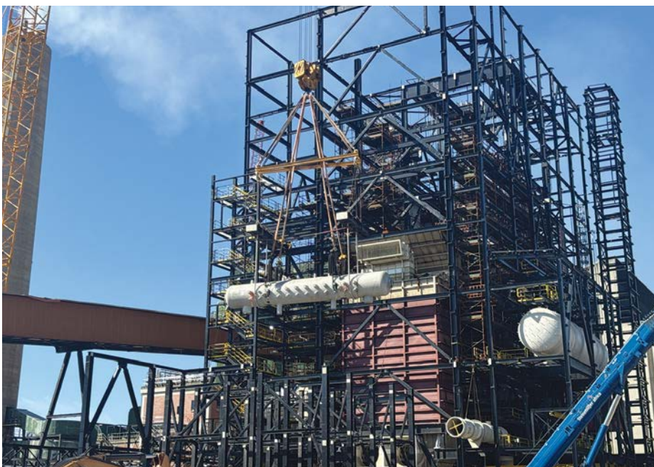
Steinmüller Africa is leading an 18-month boiler construction project for the pulp and paper industry. Shown here is the pre-fabricated steam drum, the heart of the boiler, being lifted into place.
