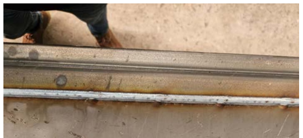
The finished weld seam is smooth with a consistent width and little spatter on the surrounding surfaces.
