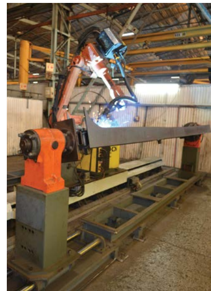
Robot welders and manipulators are typically used for long-section welding where surface finish is important.
