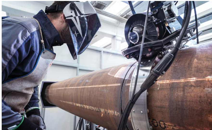
Böhler Welding's hybrid girth welding methodology uses the pipeRunner® bug and band system for fill and cap welding, with uphill progression using a conventional V-bevel joint preparation and rutile flux-cored wires.
