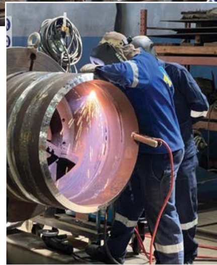
Steinmüller Africa looks for talent among the communities around boiler plants, picking up those who don't have higher qualifications and taking them from basic training and onto being A-plus welders.
