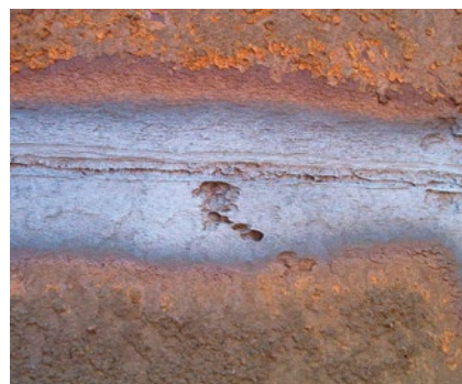
Figure 2: Stress corrosion cracking in welded joint.
