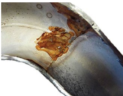
Figure 1: Crevice corrosion adjacent to a stainless steel pipe weld.
