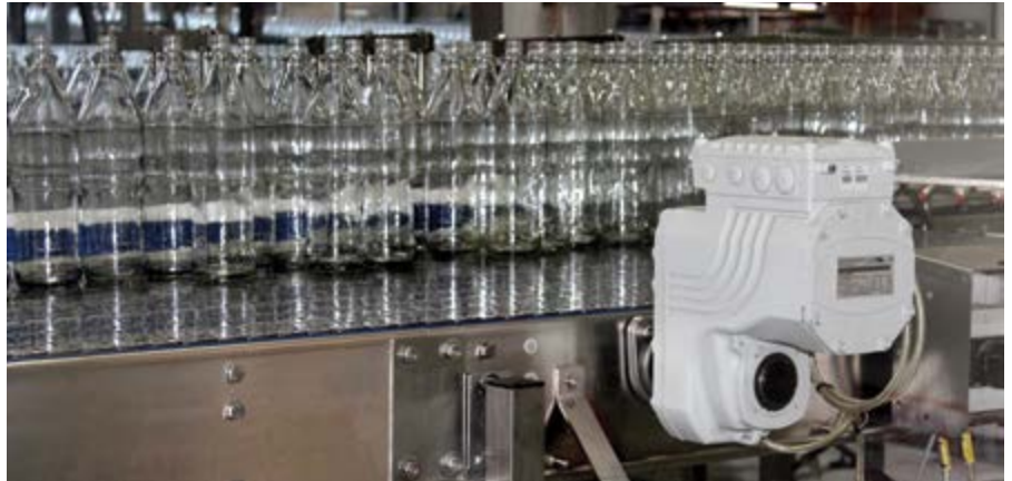
At a beverage bottling plant in Nigel, SEW-EURODRIVE has recently installed 53 MOVIGEAR units for an additional line.
