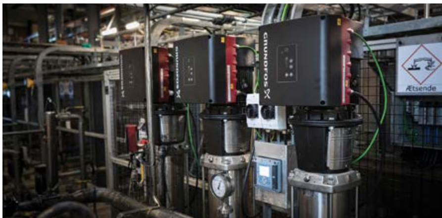
A Grundfos three pump booster set with a cascade function: when flow varies across the plant the booster set can maintain constant pressure with varying flows depending on wash-and-clean demand.
