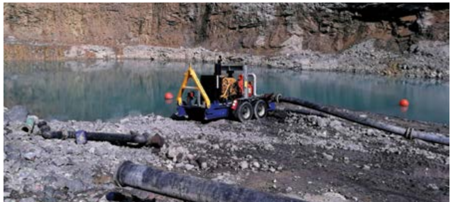
A second Sykes XH150 dewatering pump has been set to work at a mine in the Northern Cape, dewatering a flooded area at a 100 m static head pumping a distance of 1.8 km through a 250 mm pipeline.
