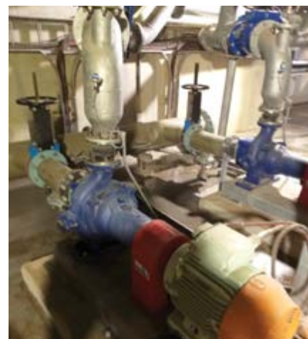
With flooded suction installations, a horizontal end-suction pump is installed below ground in a dry underground chamber.
