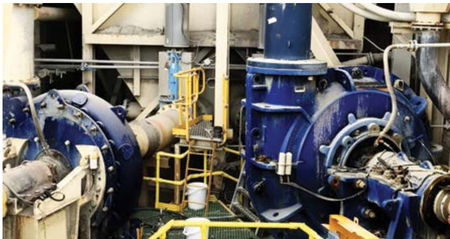
Weir Minerals improved the wear life of pumps by 140% at Evolution Mining by installing a Warman MCR 550 slurry pump.
