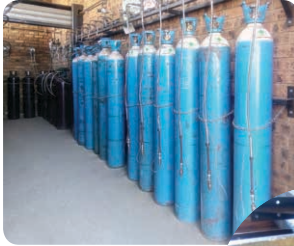
Above: Gas cylinders of Arcal Speed waiting to be connected to SE Steel Fabrication's shielding gas reticulation system.
